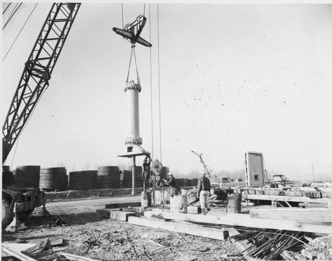
View showing method of raising slide gate hoist cylinder with 8 cy. cable & mobile crane.
