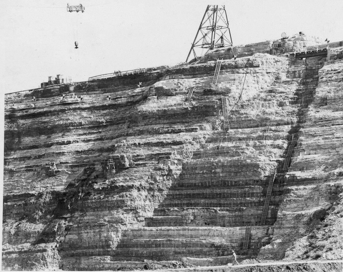
View, looking downstream and toward right abutment, showing overhang. Compare with TR-674 and 675.
