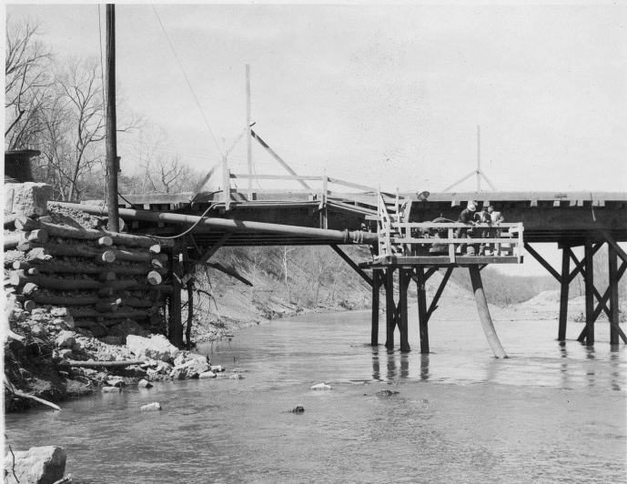
Water supply pump for No. 1 Settling Pond, looking upstream at contractor's bridge.
