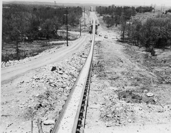
VIEW LOOKING TOWARD CONTRACTOR'S PLANT FROM ACCESS ROAD TUNNEL, SHOWING "B" CONVEYOR BELT IN OPERATION.
