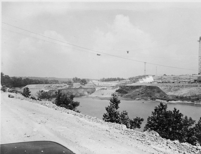
VIEW, LOOKING UPSTREAM, SHOWING DIVERSION STAGES. STAGE I COFFERDAM RUNNING PARALLEL WITH RIVER. AT EXTREME RIGHT DOWNSTREAM END EXCAVATED FOR STAGE II DIVERSION. LOWER LEFT STAGE II DOWNSTREAM COFFERDAM, UPPER LEFT STAGE II UPSTREAM COFFERDAM.
