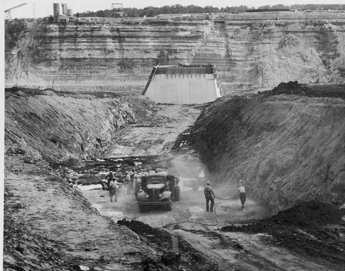
View, looking toward right abutment, showing clean-up operations in core trench at Sta. 43+00.
