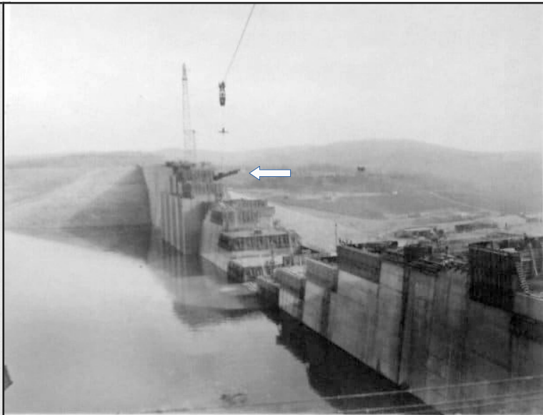
View showing 8 cy. cableway at Table Rock Dam lifting ferry push boat from lake for repairs. Arrow pointing to boat
