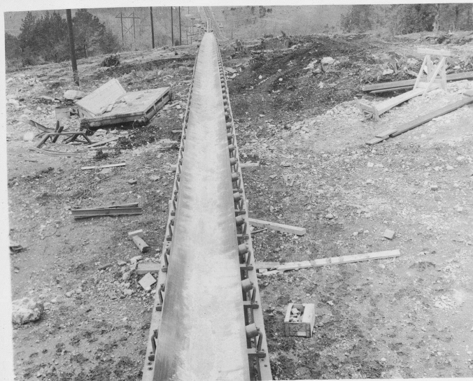
View of conveyor belt from quarry site surge pile, looking toward plant on right abutment. ( 2.8c rolleiflex. ) 18 March 1955 Table Rock TR 239
