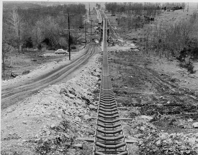
'B' conveyor belt line from tunnel to scrubber, 2-8c rolleiflex— 18 March 1955
