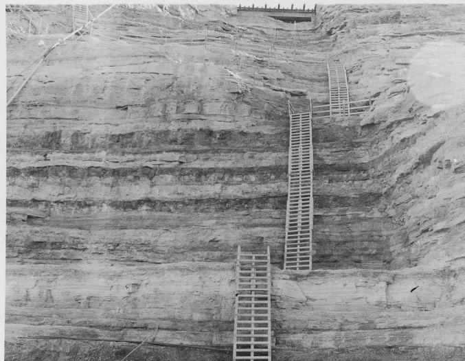
View of Keyway, Rt. Abutment Looking Along 10,00 Line Up Face of Keyway
