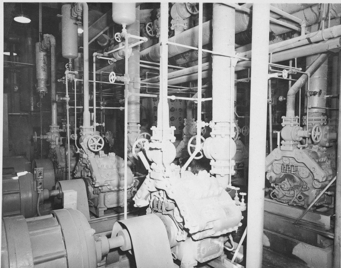
VIEW OF INTERIOR REFRIGERATION COMPRESSOR ROOM IN COOLING PLANT.
