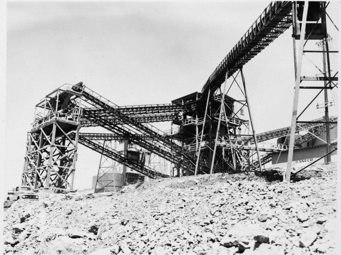
VIEW SHOWING INTER-CONNECTING CONVEYORS, ON LEFT IS TRANSFER STATION, ON RIGHT IS SCREENING PLANT.
