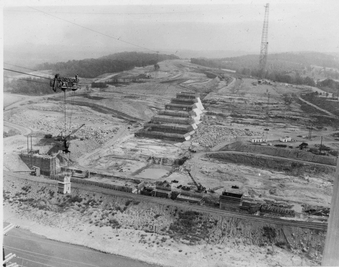
VIEW, LOOKING NORTHWEST, SHOWING PROGRESS ON MONOLITH 15 AND LEFT TRAINING WALL. AT EXTREME LEFT CENTER EXCAVATION HAS STARTED ON UPSTREAM END OF STAGE 1 COFFERDAM. 11 AUGUST 1955
