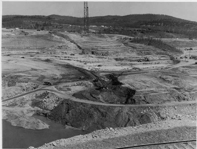
General view of left abutment from Sta. 63/01, Ra. 6/00, looking north-northeast. 30 March 1955 Table Rock TR 303
