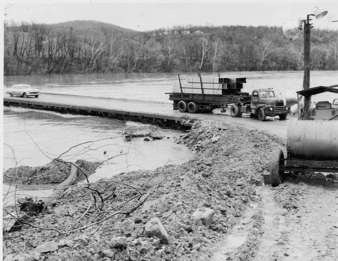
Contractor's bridge, upstream side to left embankment, river water level 23.60, 2-8c rolleiflex.
