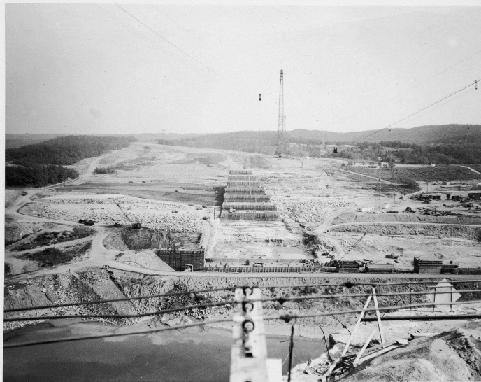
View, looking along axis of dam from right abutment, showing progress on Monolith 15 and left training wall.
